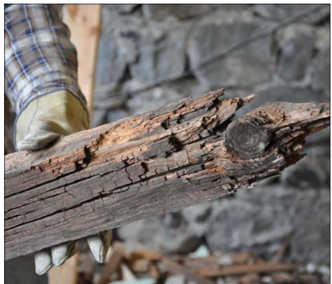
Exhibit A-Rotten wood.
